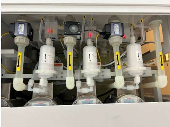
SAC Filter Rack
